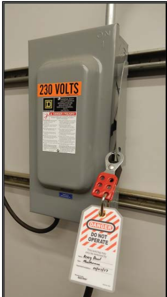
Figure 1: Lockout/Tagout on the Power Source Panel
