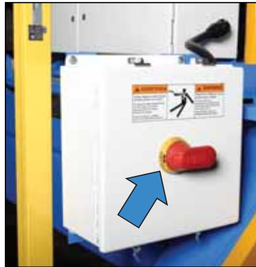
Figure 3: Disconnect Switch to Lockout/Tagout
