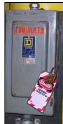
Figure 2: Lockout/Tagout on the Power Source Panel
