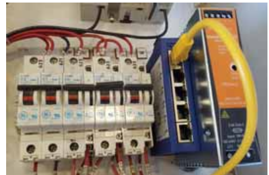
Figure 19: Yellow Cable Entering the Ethernet Switch
