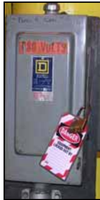
Figure 1: Lockout/Tagout on the Power Source Panel
