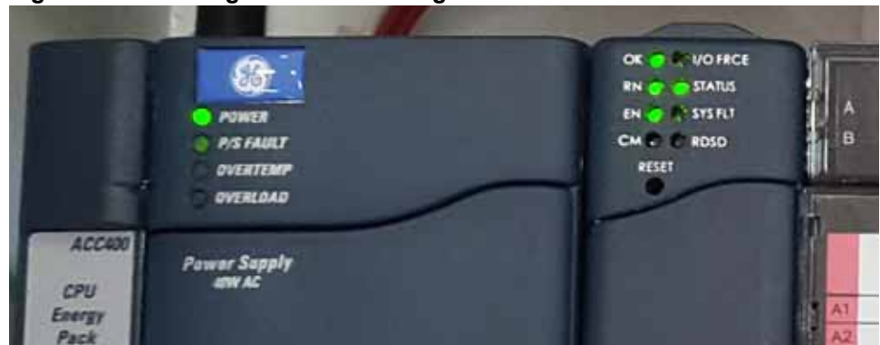
Figure 21: Checking PLC Indicator Lights
