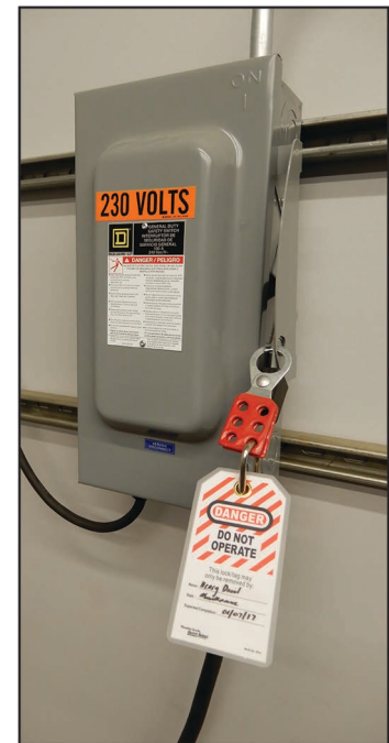
Figure 1: Lockout/Tagout on a Power Source Panel
