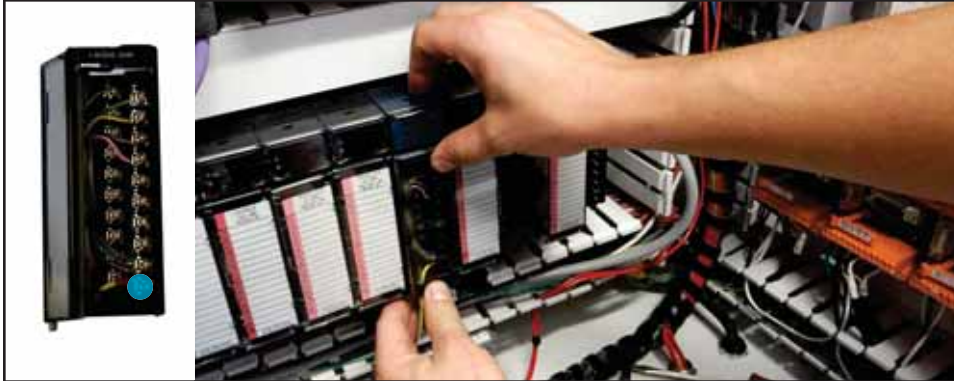
Figure 29: Connecting Analog Output Module End of the PAC
