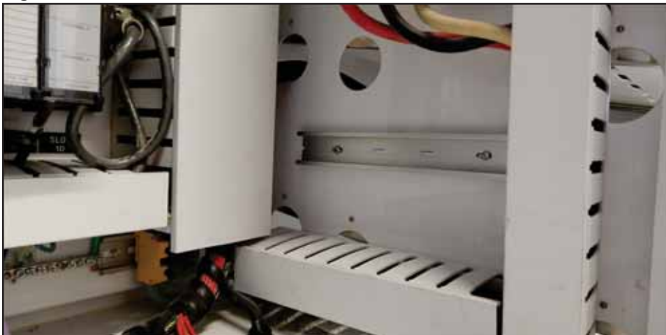
Figure 15: DIN Rail Mounted to Electrical Enclosure Wall
