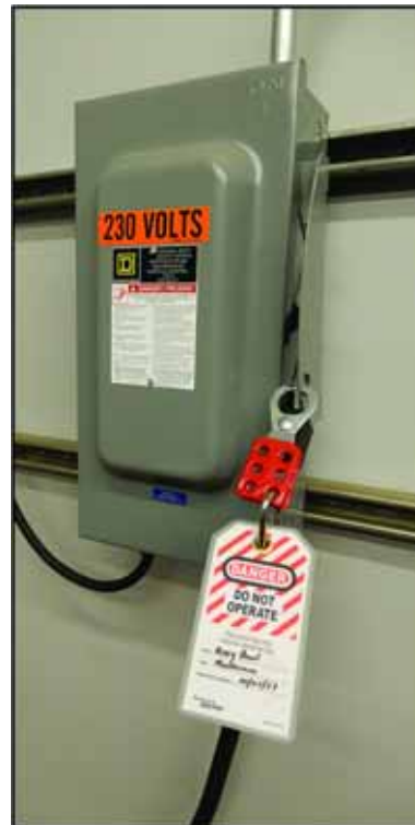
Figure 13: Lockout/Tagout on the Power Source Panel
